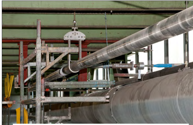
Pipe with support construction
